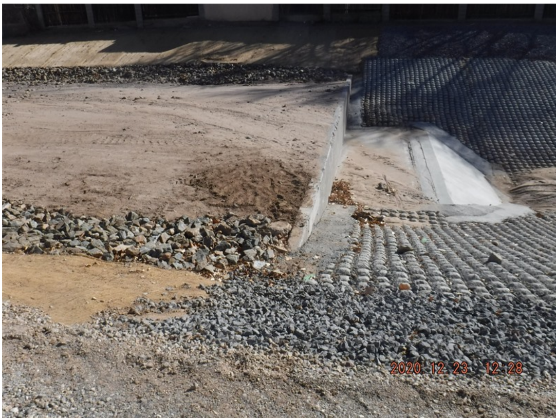
Photo facing south, Car - 5: Formwork for grade control structure extension removed by Contractor AUI.
