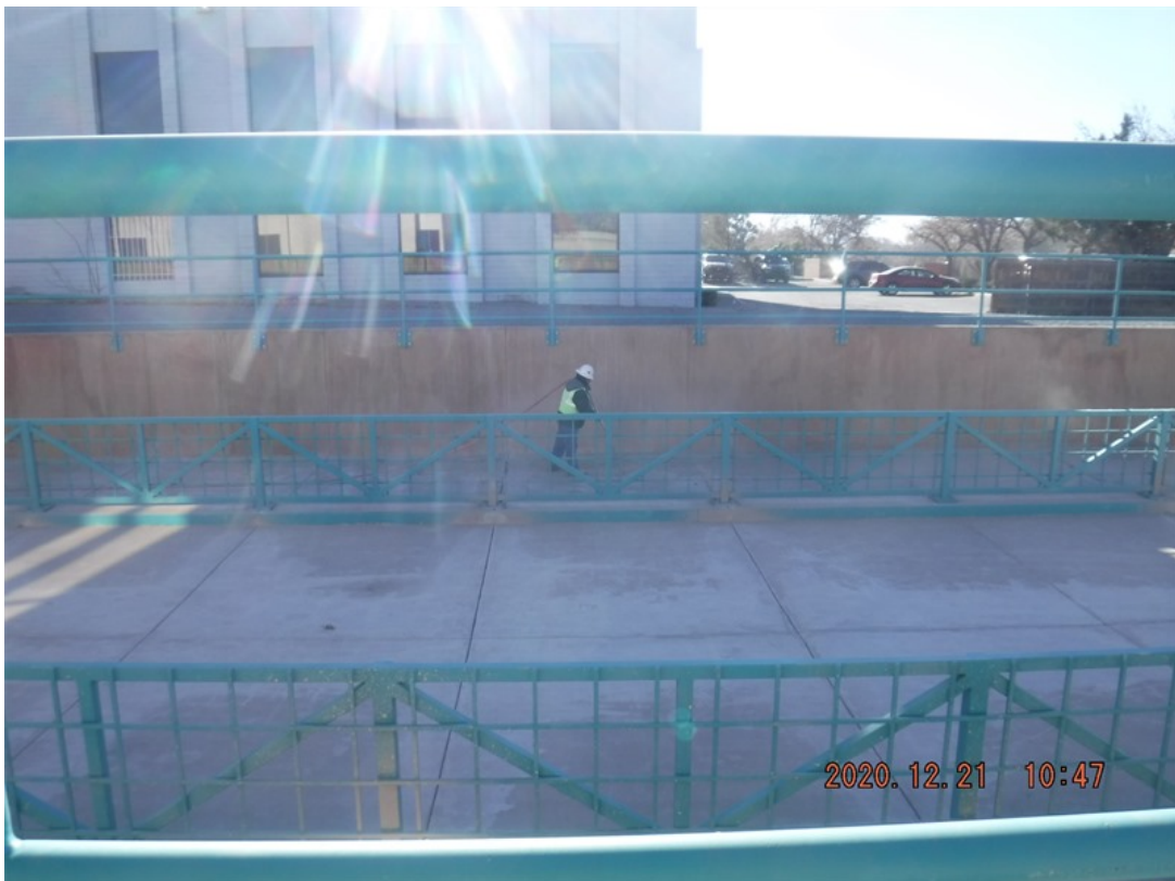
Photo facing south, Car - 1: Contractor AUI cleaning out control joints to prepare for sealant.
