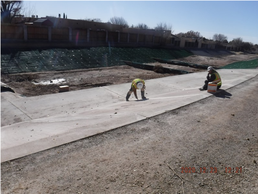
Photo facing southwest, Car - 1: Contractor AUI applying primer to construction joint to prepare for sealant.
