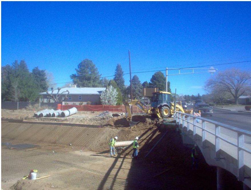
RMCI compacting around pipe penetrations Iron workers will be able to tie rebar together over these areas tomorrow
