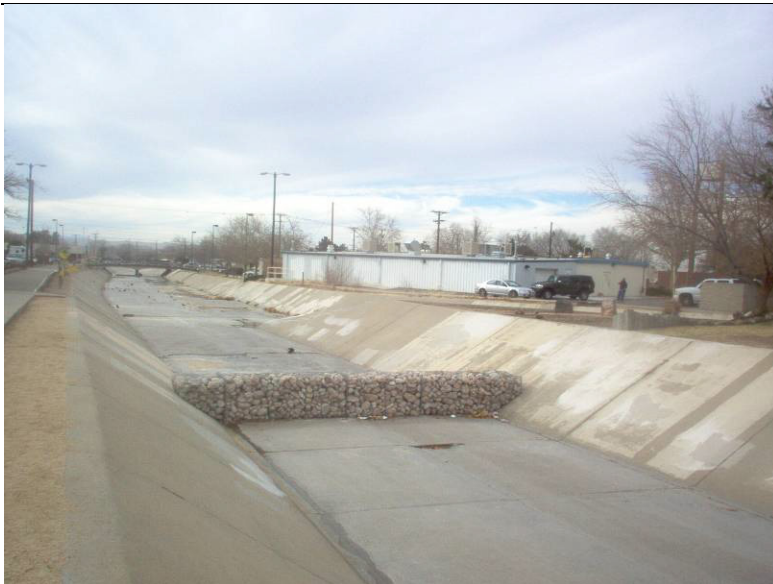
Gabions across the Hahn Arroyo placed above the confluence for the SWPPP.
