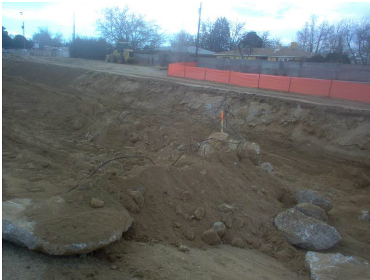
North side of the channel 25+00 to 26+50 +/- at 25' Left, contractor encountered an existing headwall and asphalt paving.
